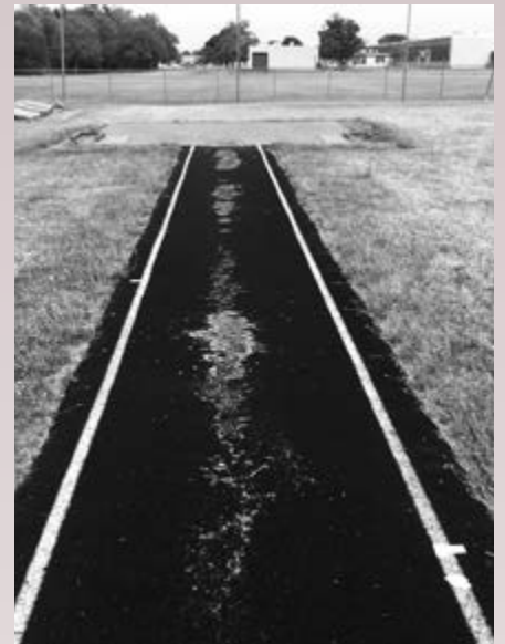
Worn out all weather track long-jump runway
