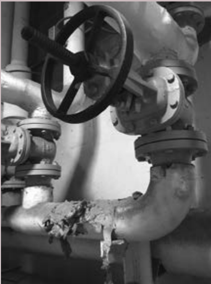
Deteriorated piping at the high school
