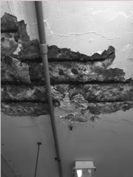
Disintegrating concrete at pool
