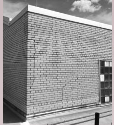
Masonry work needed at pool wall
